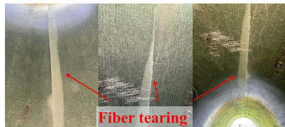
Fig. 19. Failure Cracking of the CIPP Liner.
